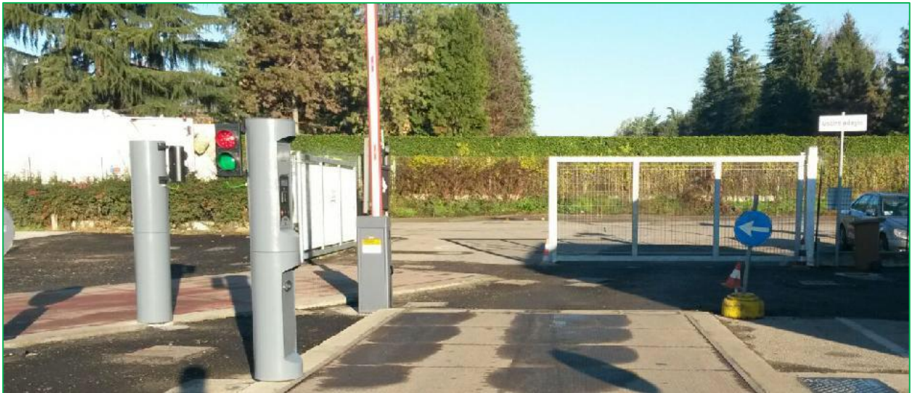
EECO Check installation example in a waste collecting area. In evidence: the weighbridges and the totem.
